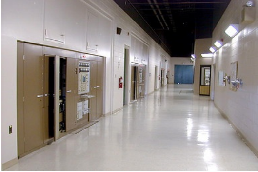
4x500kW Tx Hall
