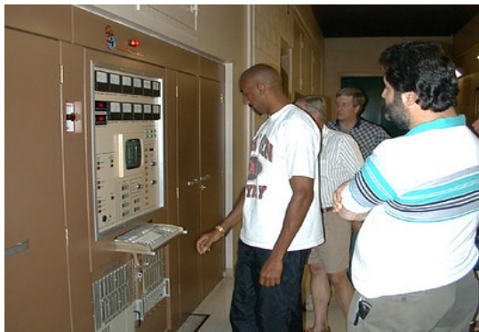
4x500kW Tx Front Panel
